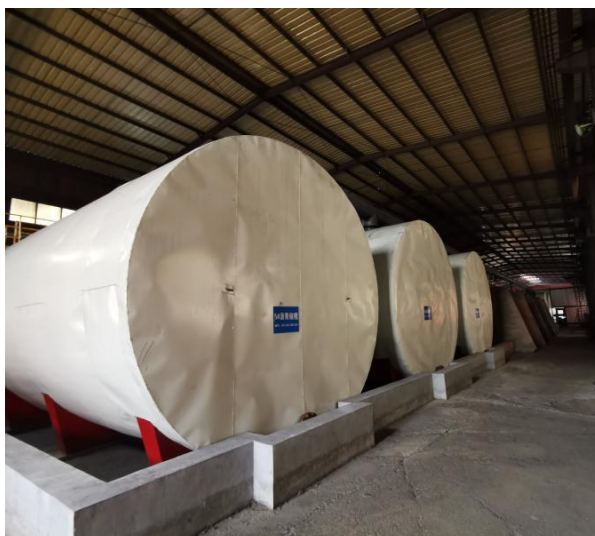
沥青储罐，置于围堰
